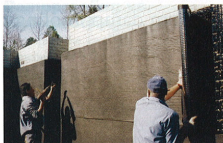
■ With wall insulation there is less likelihood of thermal or air leakage.
