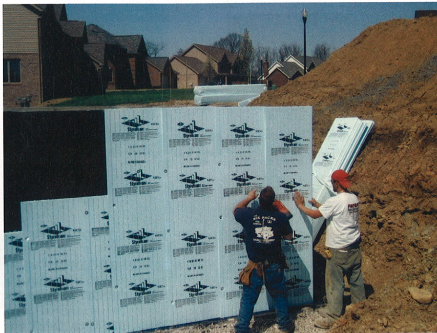
■ Insulating the exterior basement wall during new home construction protects the waterproofing membrane.
